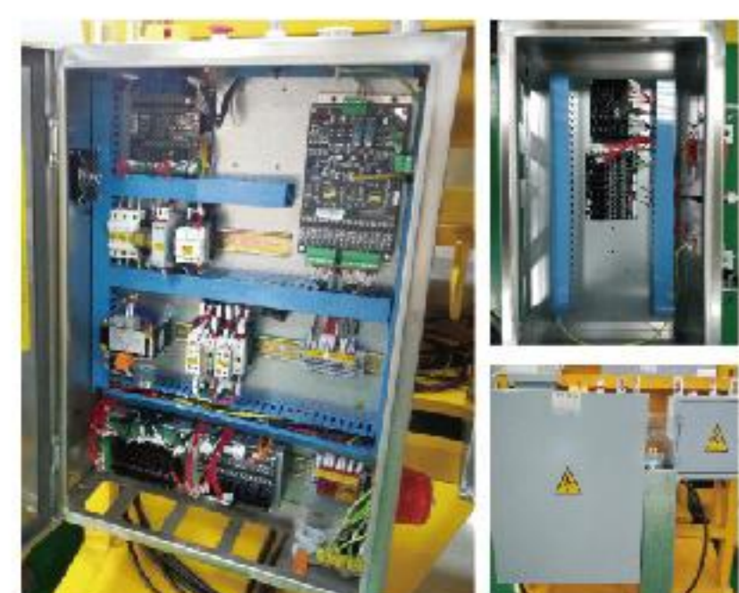
·Escalator control cabinet
